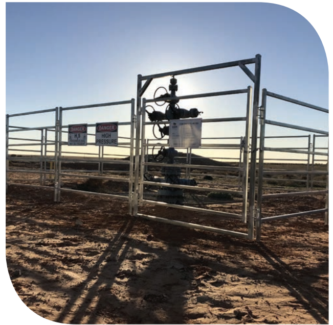
Image: Fencing around Halifax-1 wellhead
